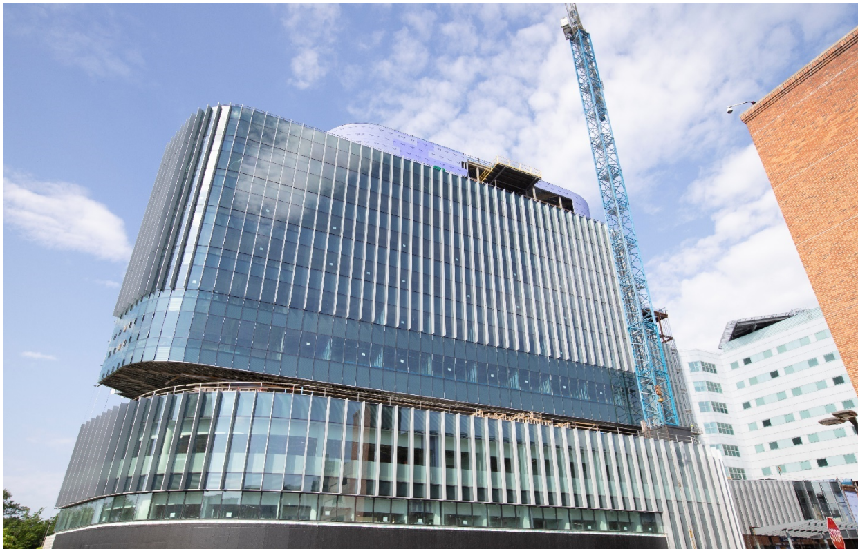
Figure 6: The University Hospital Expansion project, where our office is using innovative inspection methods
