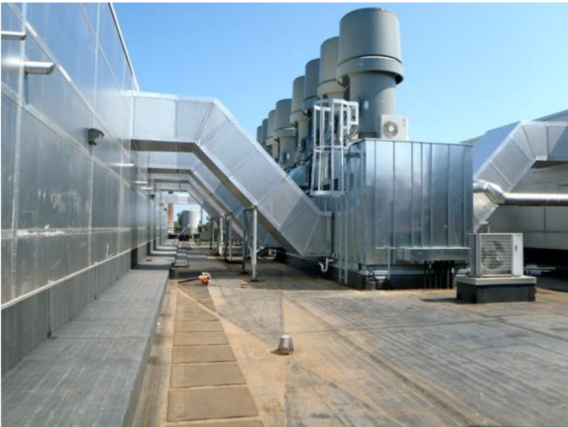
Jordan Hall Exhaust Systems – October 5, 2012
